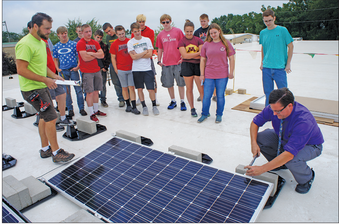
Construction of Juda School District's new solar array began on Tuesday and Juda High School students got a first-hand look at the solar installation process.
