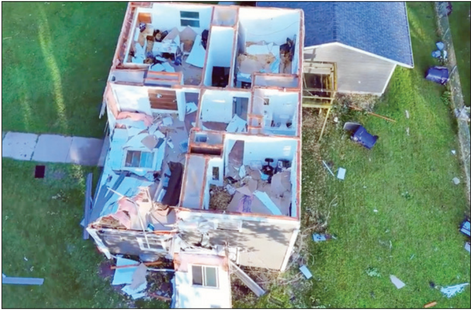
PHOTO COURTESY CHICAGO AND MIDWEST STORM CHASERS Rock Valley Publishing A home received a lot of damage after a tornado moved through Janesville on the evening of Saturday, June 22.
